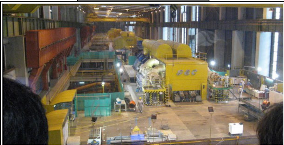
A view of the power generators at the CLP power plant showing the three generators.
